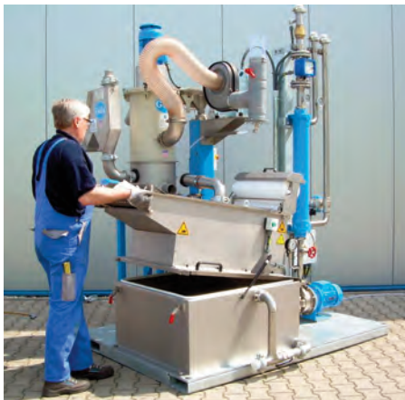
Tempered water system with band filter
