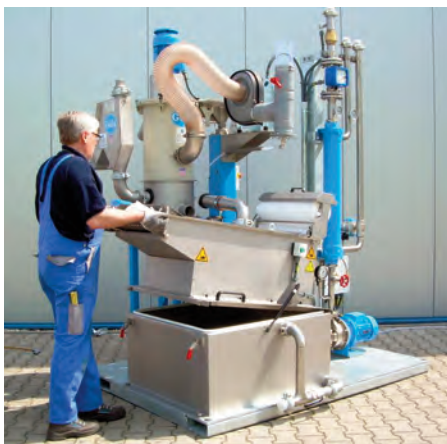
Tempered water system with band filter
